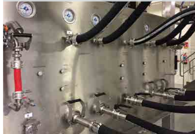
Transfer panel for raw material introduction and sample taking with cleaning in place of hoses and rods
